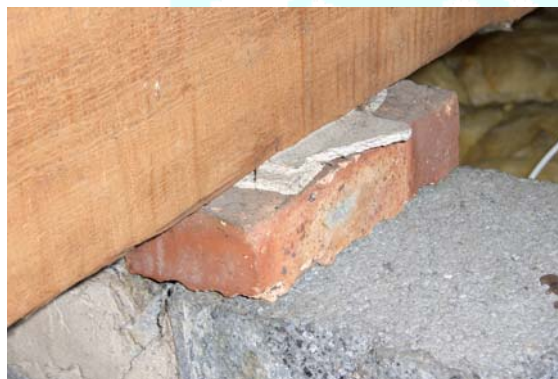
Asbestos Insulating Board ("Asbestolux") used as packing.
