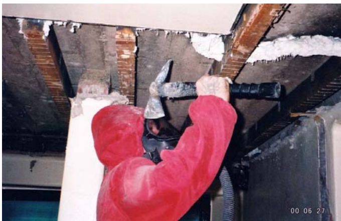
Dry stripping – please pass the Prohibition Notice!
