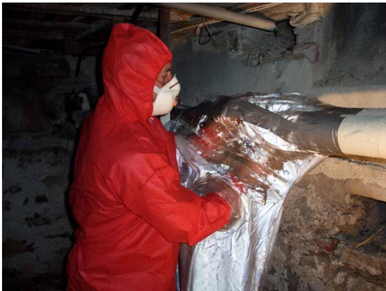
Using a glovebag to repair a leaking valve on an asbestos lagged pipe
